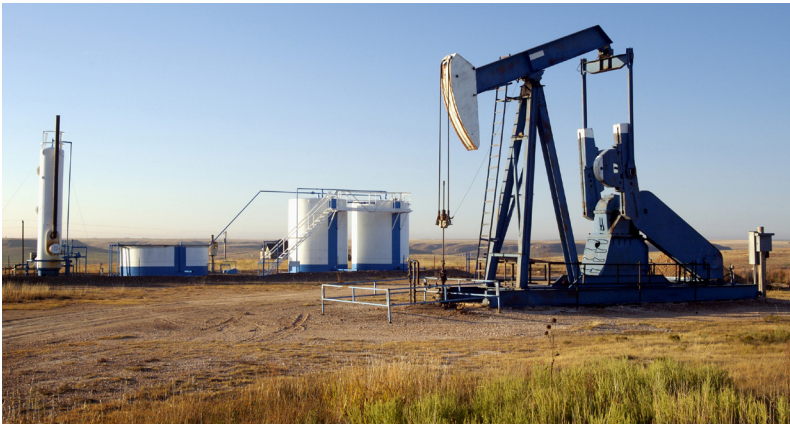
Figure 3. A well pad with associated tank battery. The tank battery holds the crude oil/water awaiting transport to a refinery. SignalFire wireless equipment is used to monitor and control various well pad automation points, including tank level.
